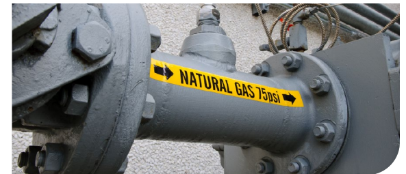
▶ Pipe markers and valve tags
